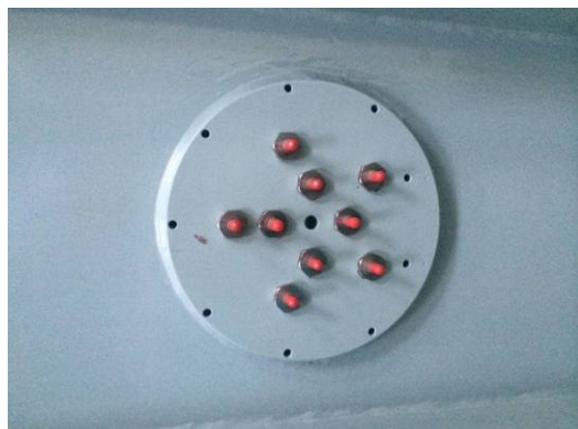
Fig. 6 Fiber-optic pressure sensor installation location and transfixion device.
